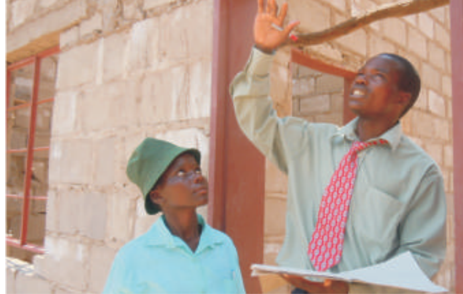
Elen Mumpande a school pupil (left) and the deputy head for Sinasengwe Satellite School, Lovemore Muzamba at the new classroom block site.
