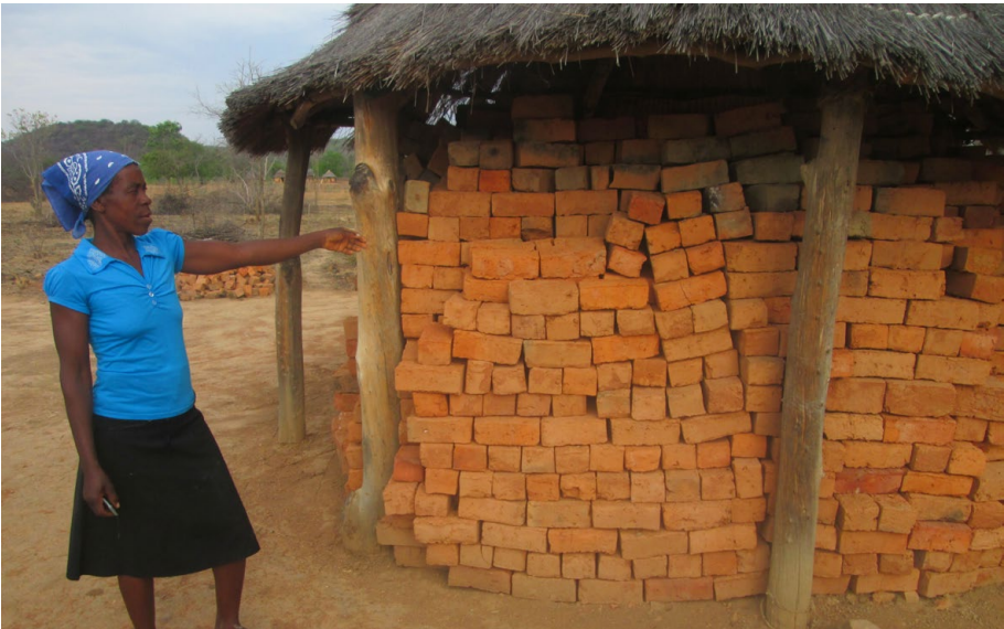
Egness Muleya of Kububa, Binga pointing at bricks her community has moulded towards the building of a clinic in the area
