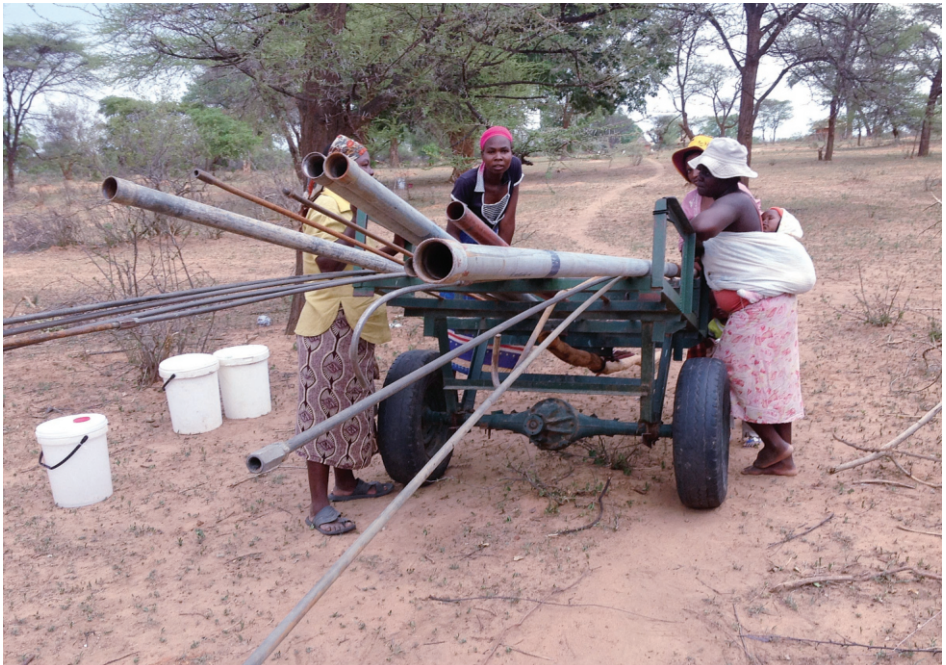
Women from Nkayi carry pipes for the repair of a borehole in their area
