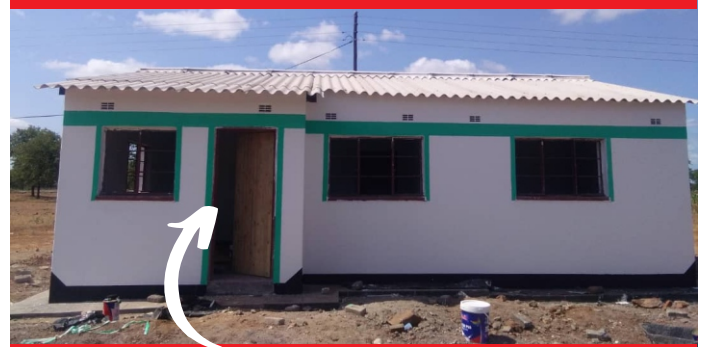
Teclar's new house constructed by AAZ and partners at Chitepo Primary School.
