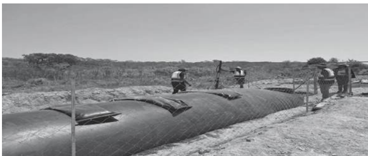
Figure 1. Prefabricated biodigester installed by Lanforce Energy in Matabeleland North
